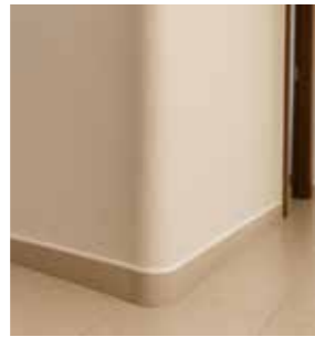
Rounded edge walls for safety
