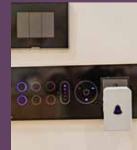
Light control switch box from FFL to bottom of switch control
